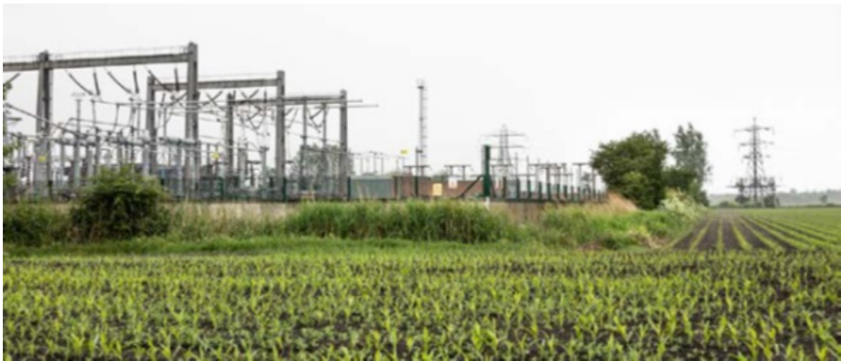
Burwell substation, location of one of Corcel's FGS projects. Source: Company
